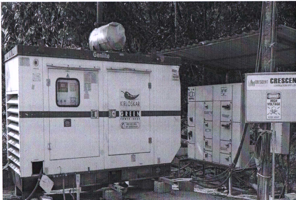
The Photographs of DG set using for construction work with the acoustic enclosure.
