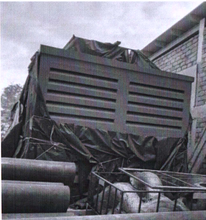
The Photographs of the acoustic installation works of DG for the project
